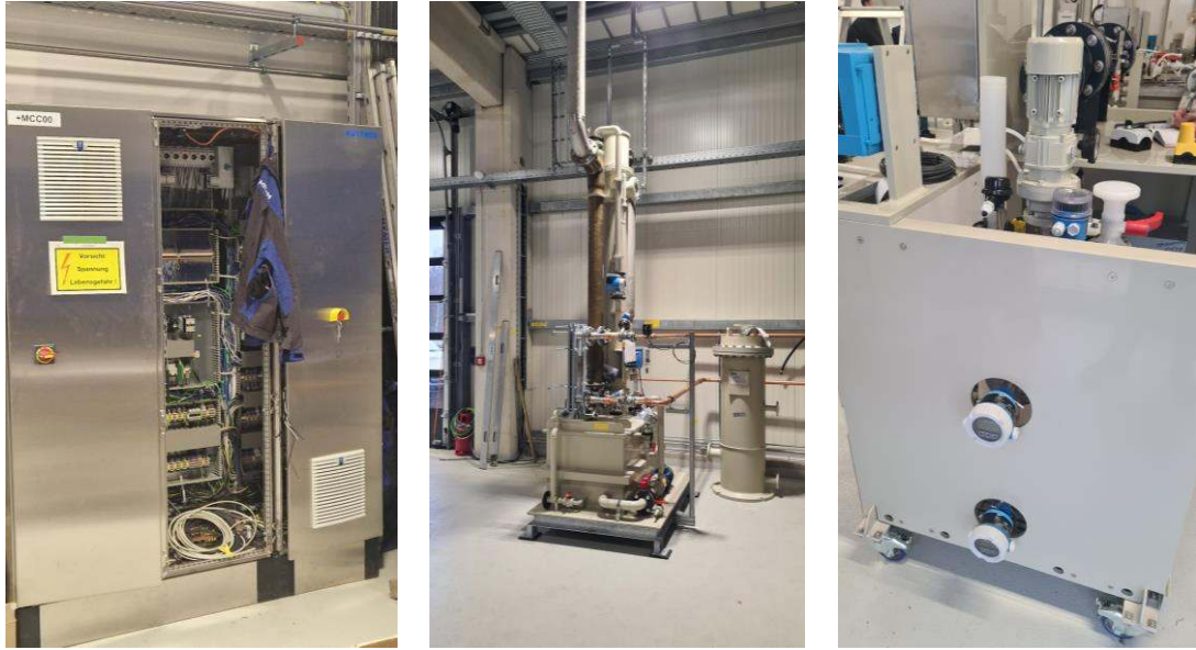
Figure 4 – Electrical Board and Various Equipment
