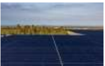
50MW Kidston Solar
