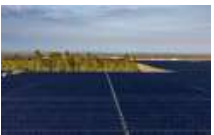
50MW Kidston Solar
