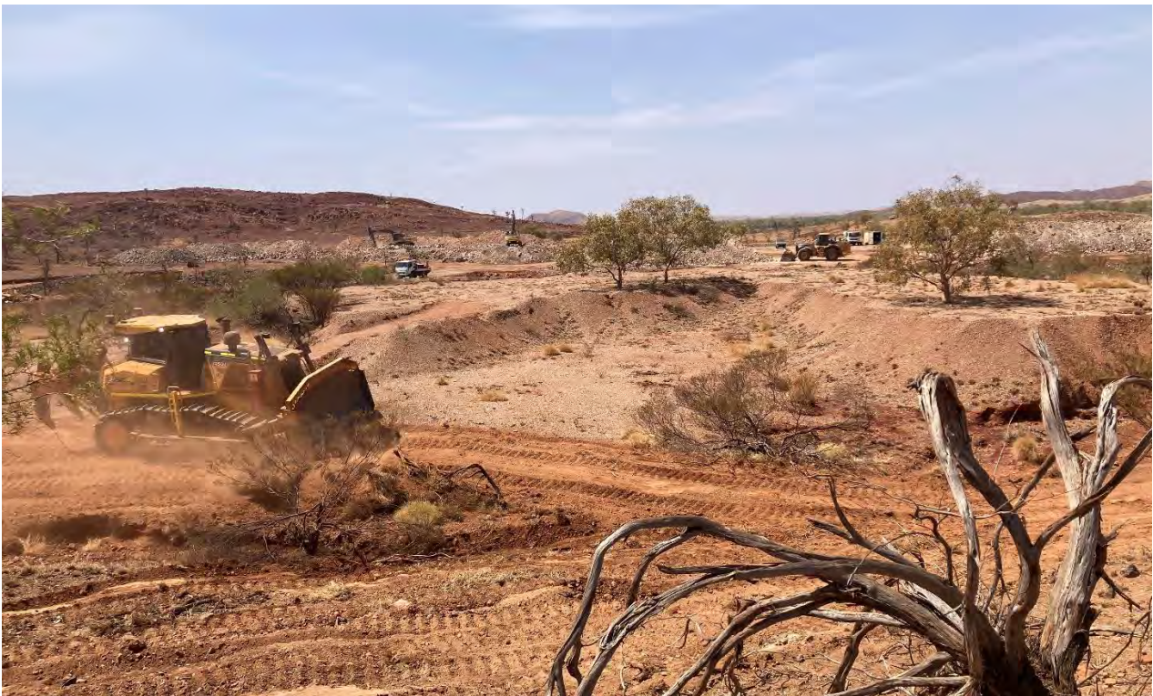
Figure 2: Clearing of Blue Bar waste dumps, with stockpiles in background and laydown yard
